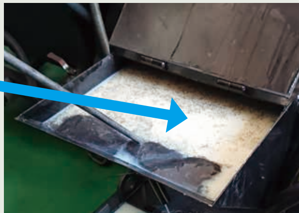
Sludge in the tank that was collected by the large flow low pressure unit.
